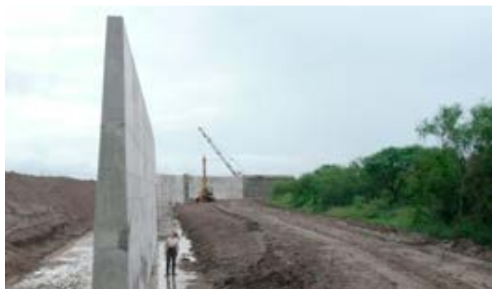
LEVEE BORDER WALL DURING CONSTRUCTION THROUGH THE LOWER RIO GRANDE VALLEY NATIONAL WILDLIFE REFUGE. PHOTO: MATT CLARK
